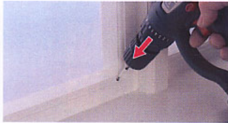
a2. Mark position as outlined in step 8 (over leaf). Drill Ø4mm hole to depth of 10mm
